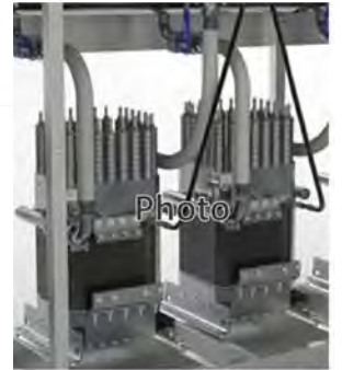
Electrolyzer Cell Stacks
