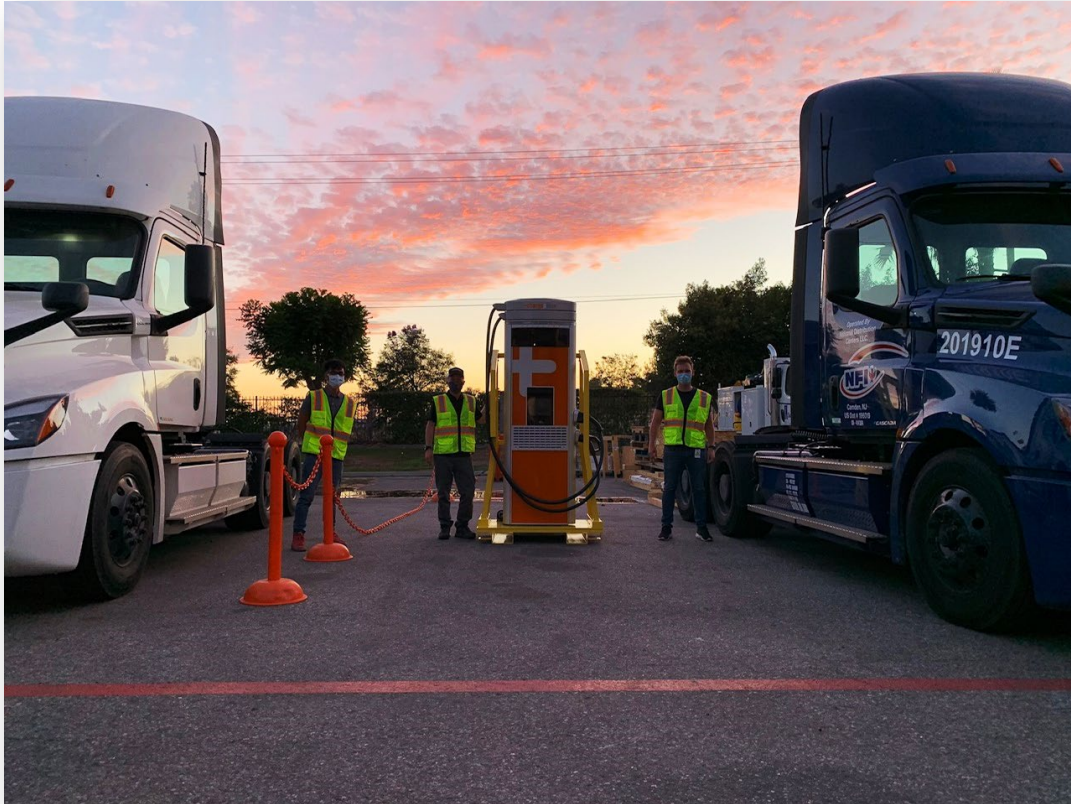
Commissioning charger in Fontana, CA. June, 2020
