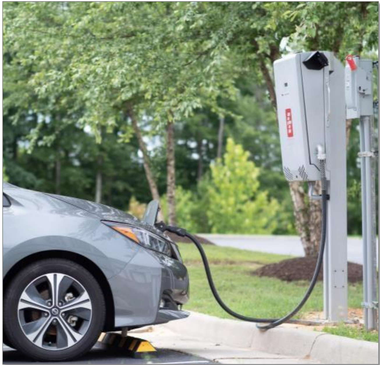
Nissan LEAF connected to Fermata Energy's FE-15 15kW bidirectional charger as part of a V2X project at the EIT manufacturing facility in Danville, VA, the FE-15's production site.
