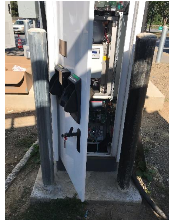
Charger with poorly placed bollard limits service entry
