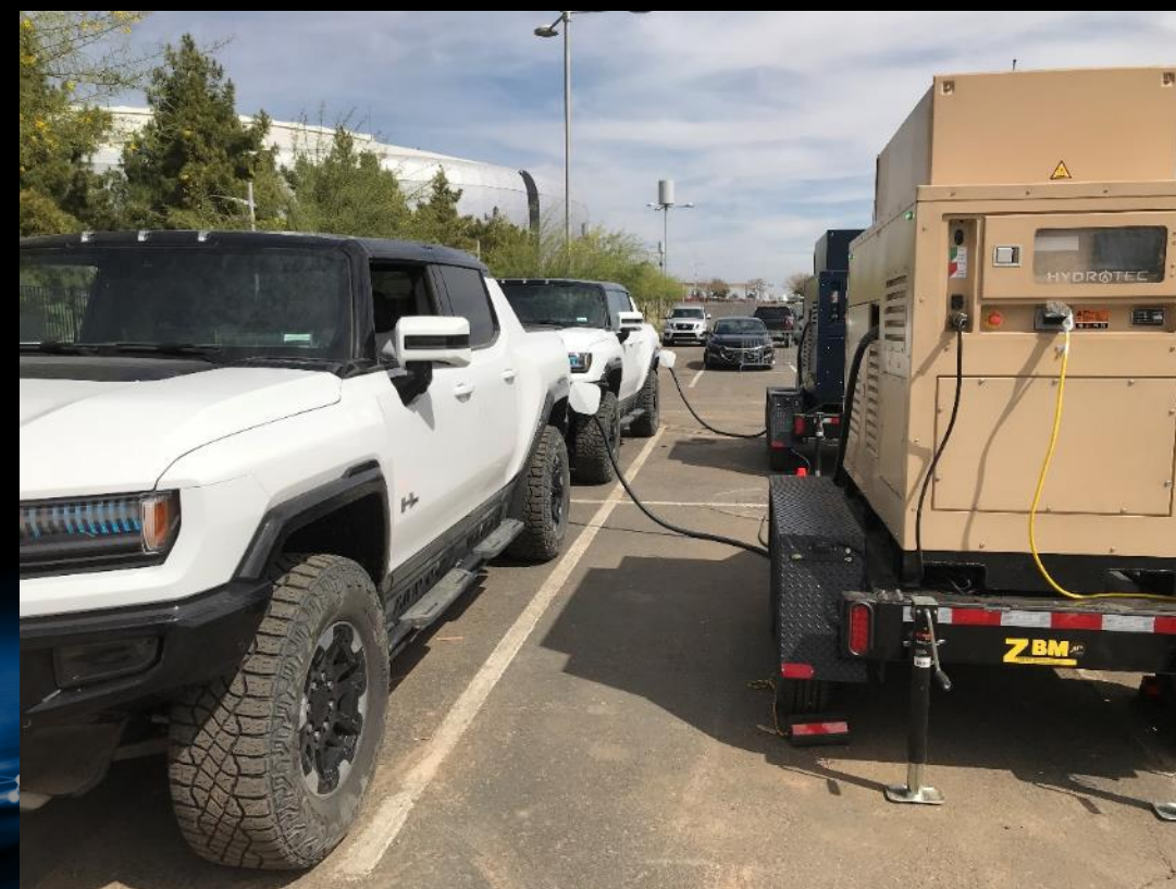
Charging Hummer EV's with GM Palletized Fuel Cell DC Fast Chargers
